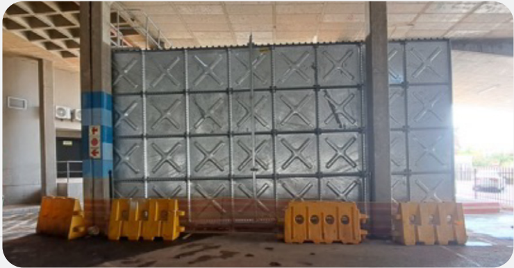
Clearwater, Hyde Park Corner and Woodlands, Gauteng, South Africa Three-day potable water backup tanks
